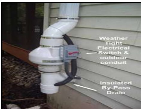
Vapor mitigation system that vents vapors to the outdoors.
