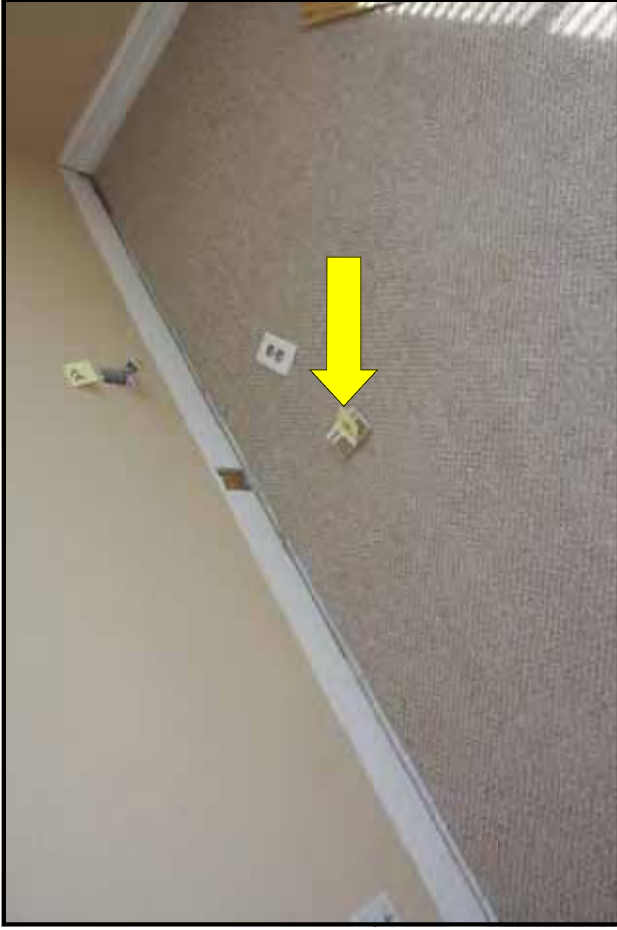
Took sample #23 from here behind baseboard. Yellow arrow points to edge tape with blue coloring. Many types of drywall have blue coloring including Knauf and BNB. Not a large enough sample to make a definite determination from the edge tape.
