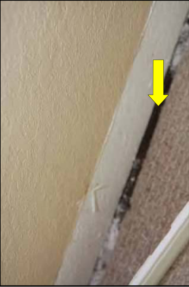
Water damage underneath that could contribute to tarnished copper.
