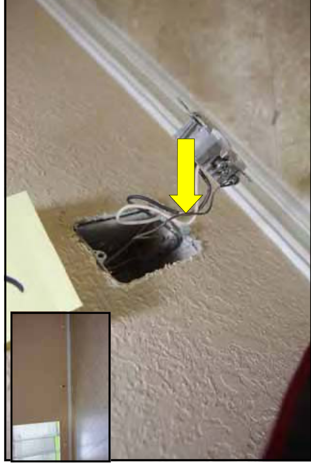
Took sample #5 from here. Copper ground wire is tarnished.
