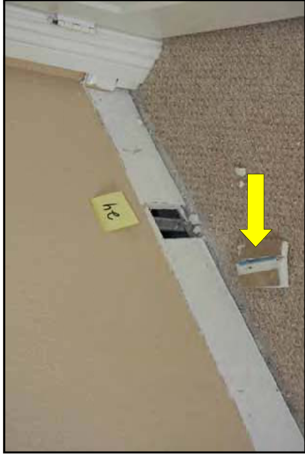
Sample #24 Removed drywall from behind baseboard to check edge tape for drywall ID. Yellow arrow points to edge tape with blue coloring. Many types of drywall have blue coloring including Knauf and BNB. Not a large enough sample to make a definite determination from the edge tape.
