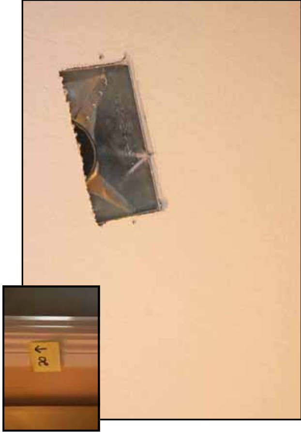
Took sample #20 from ceiling. Looks like 5/8" material which would not be problem Chinese dry-wall.
