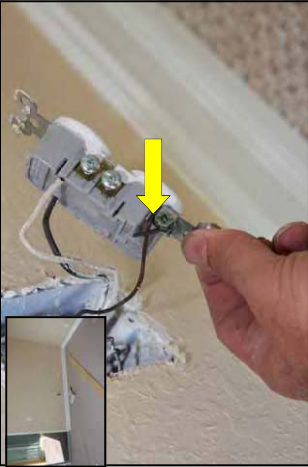
Took sample #10 from here. Copper ground wire is tarnished.
