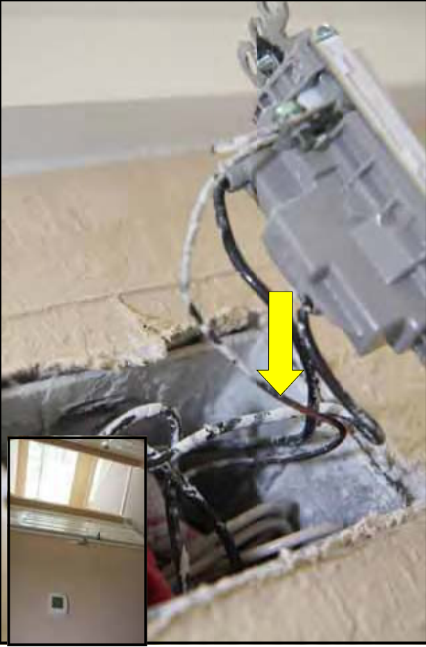
Took sample #11 from here. Copper ground wire is tarnished.
